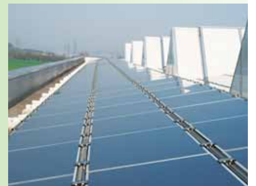
Fotovoltaikanlage. Photovoltaic facility.
